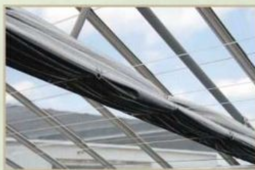
Motorized shades make controlling light a cinch.
